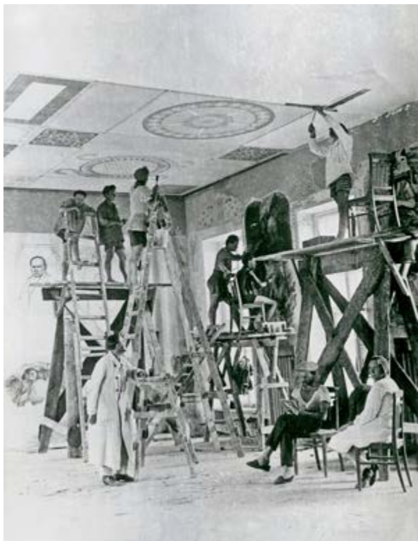
Slikanje rustikalnog lječilišta na Hadžibegovu limanu pokraj Odeše; M. Bojčuk stoji ispod skele, A. Ivanova i V. Sedljar sjede, a M. Rokicki, M. Šehtman i O. Bizjukov su na skeli, 1928. Ljubaznošću Ivana Melničuka, Kijev. / Painting of the rustic health resort at the Khadzhibey estuary outside the town of Odesa; M. Boichuk is standing underneath, A. Ivanova and V. Sedliar are sitting, and M. Rokytsky, M. Shehtman, and O. Biziukov are on the scaffolding, 1928. Courtesy of Ivan Melnychuk, Kyiv.
